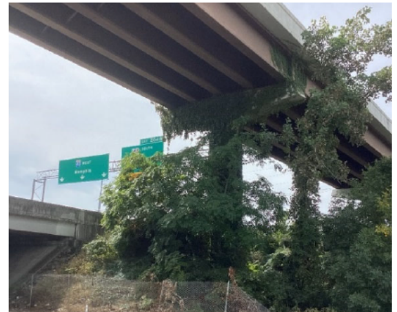
Figure 19 - Briley Parkway off-ramp from I-40 West-bound with overgrown vines and vegetation
