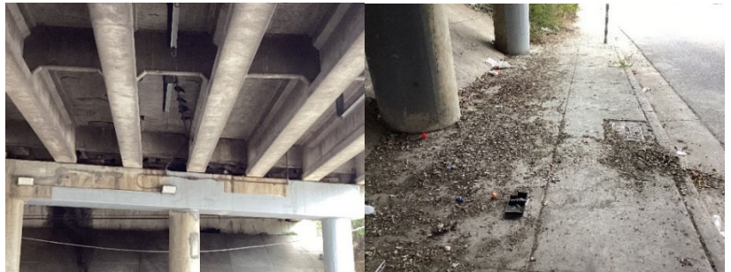
Figure 17 - Birds underneath I-40 at Fairfield Ave and bird excrement on sidewalk
